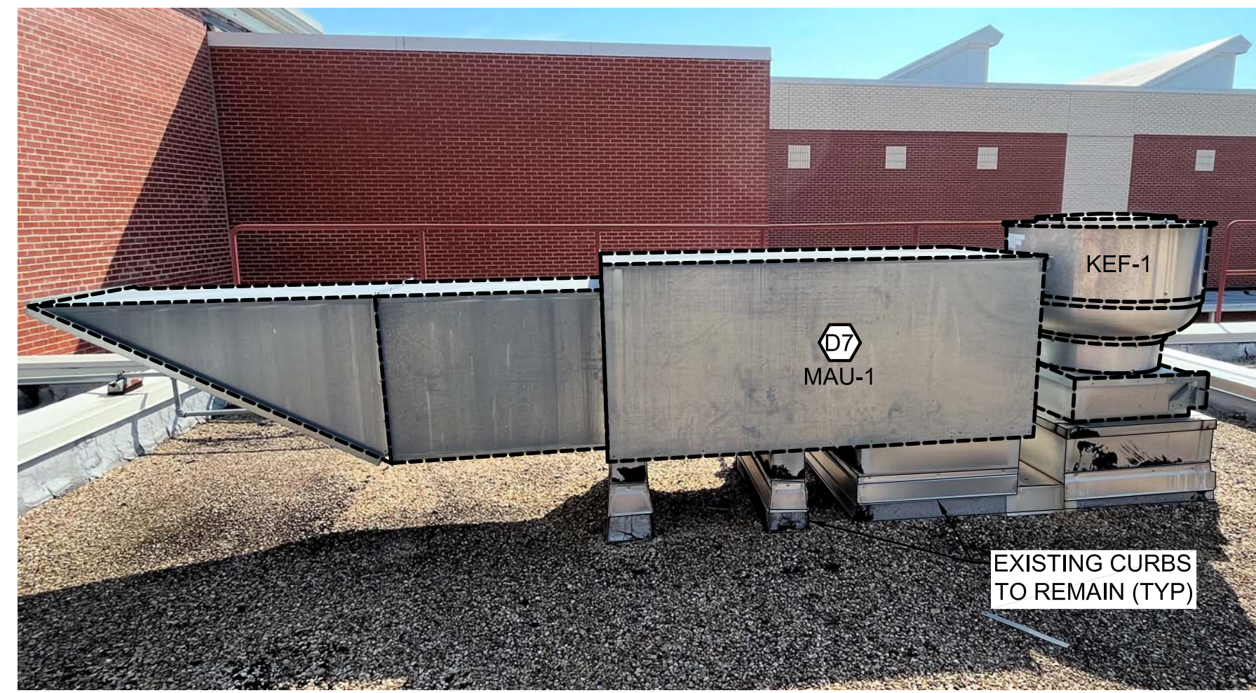
PHOTO 2 - KITCHEN MAKEUP AIR UNIT AND EXHAUST FAN EXISTING CONDITIONS.
